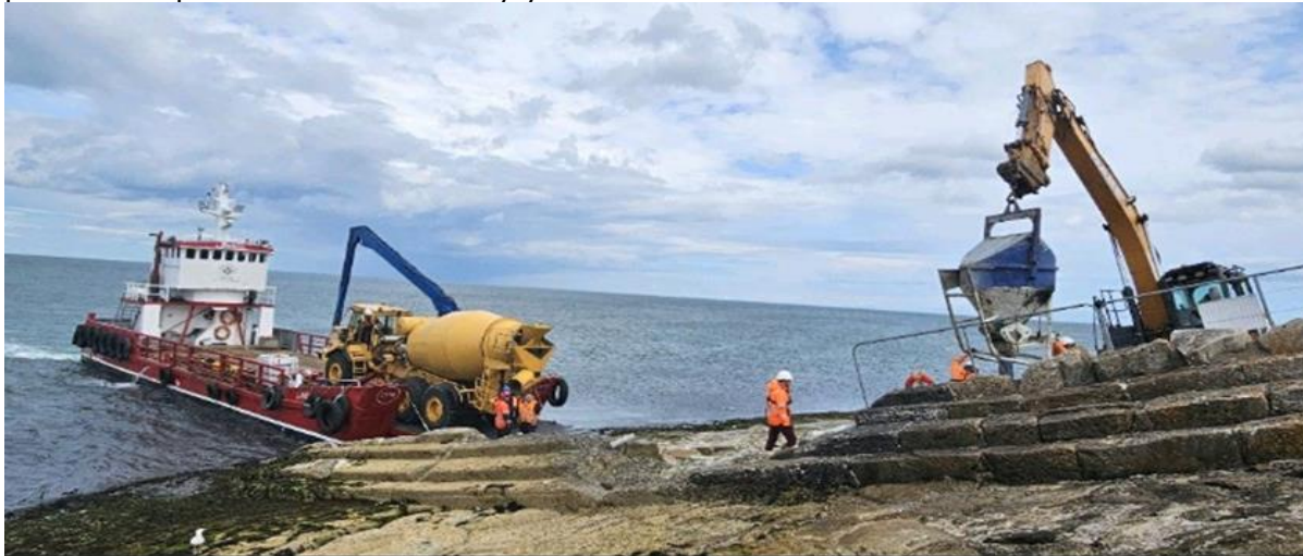
A "landing craft" delivering concrete to the back of the East Pier.
